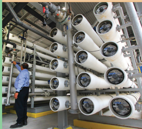
The microfiltration/reverse osmosis system at the CAWD plant transforms treated wastewater into high quality recycled water for golf course irrigation.
